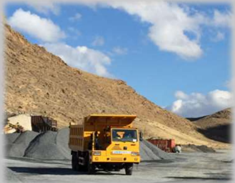
中东项目施工现场。 Construction site of Middle East mining area project.
